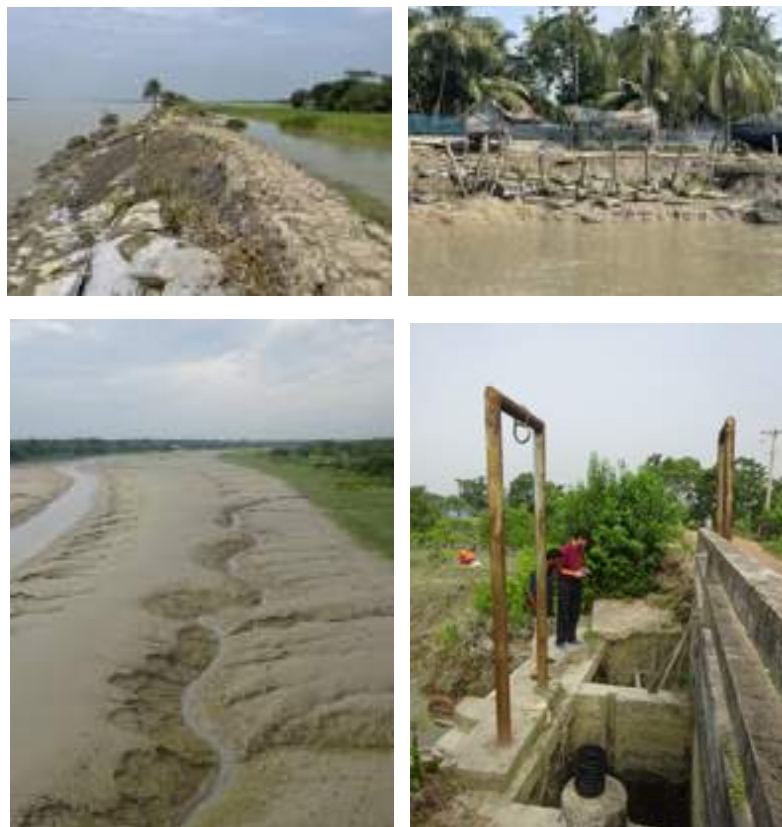
Figure 3: Fieldwork undertaken in Polders 30, 31 and 31-part, in Khulna (photos taken by authors in October 2023). The photos illustrate some of the challenges in in-polder water management.
