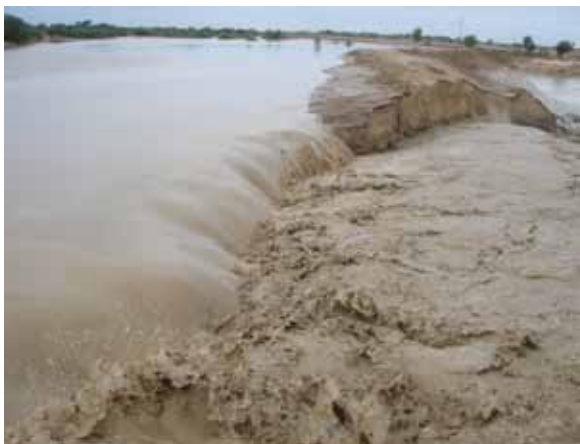
1.2 Breaking of Soil Diversion Bund
