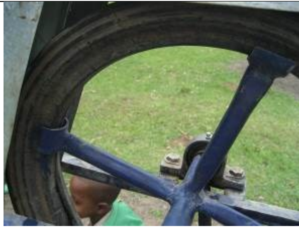
Wheel with 4 Spokes of GI pipe. Clamps in between are missing
