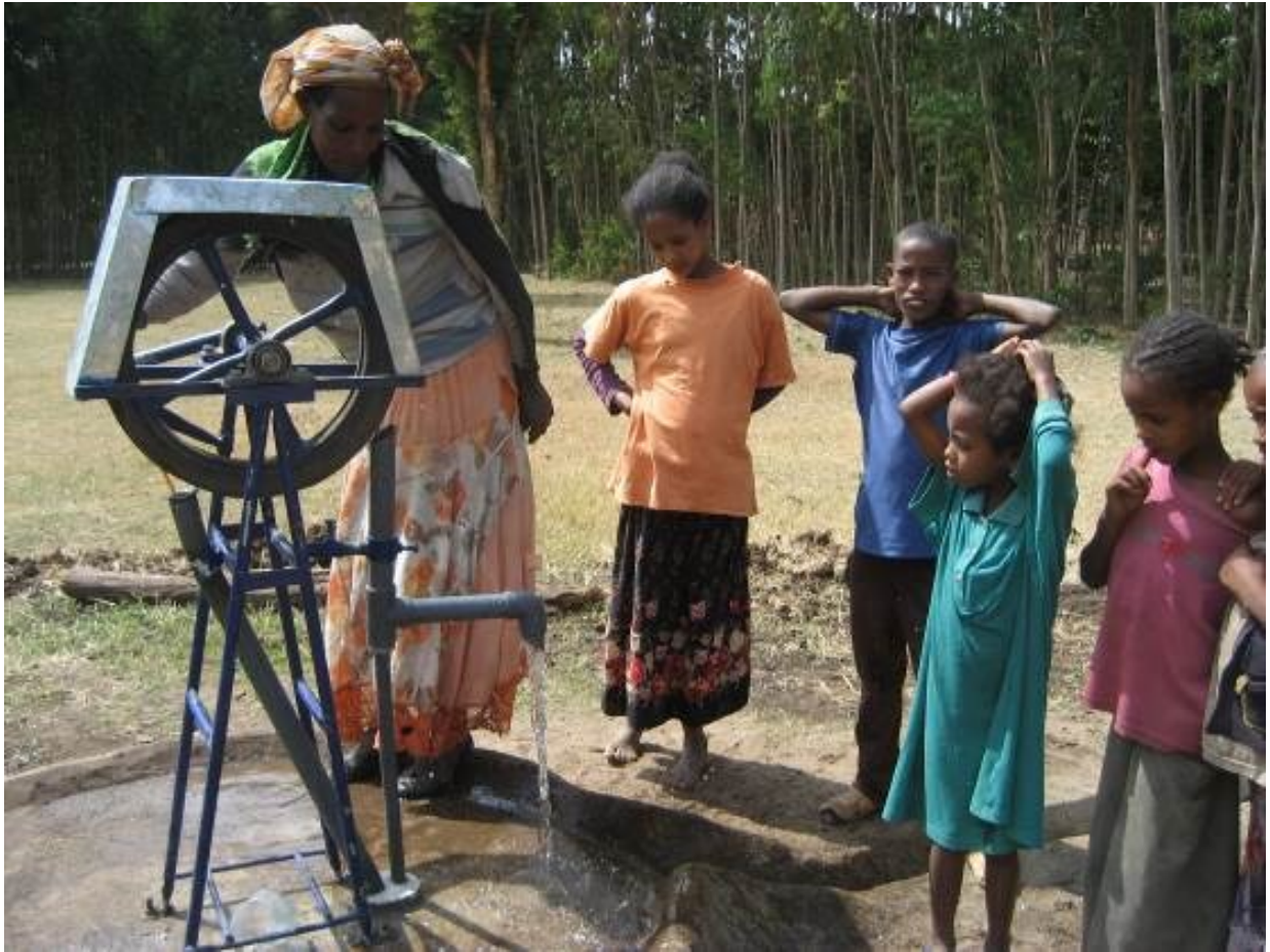
Improved Rope pump model installed in Butajera
