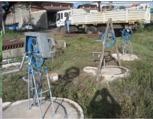
3 pump models installed at the EWTI
