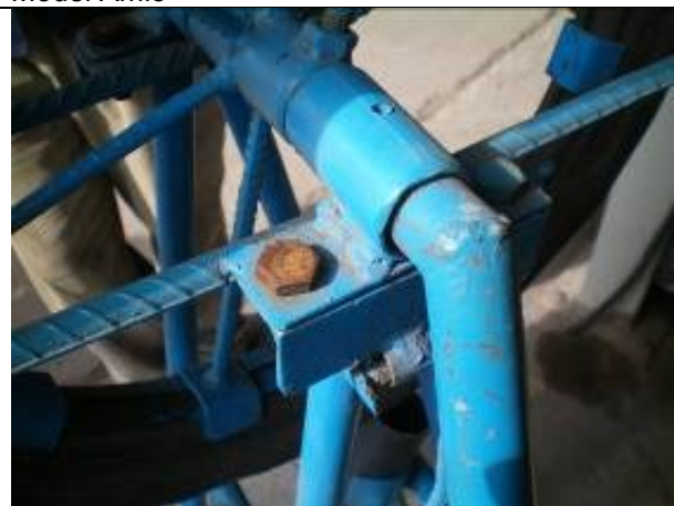
Use of black bolts instead of galvanised bolts
