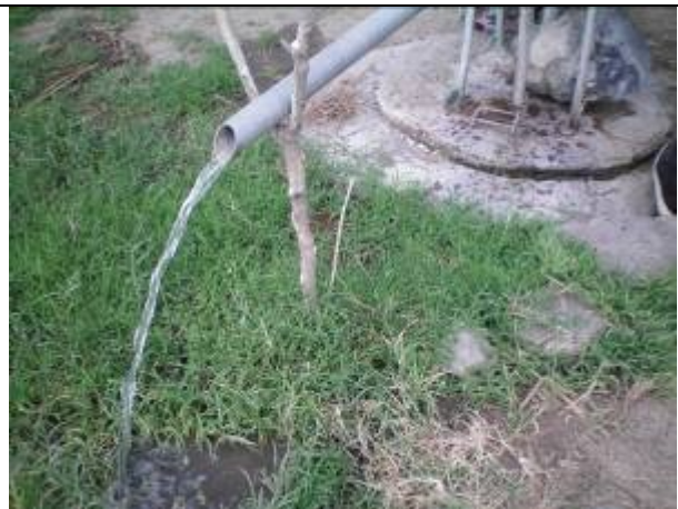
Lack of soak pit so water around the well
