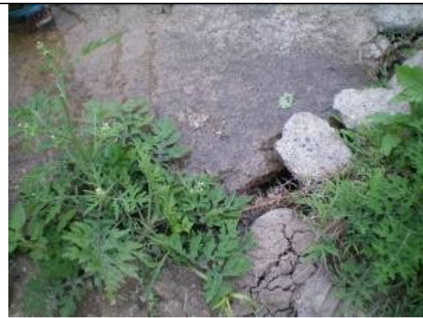
Lack of apron so water leaking back in well
