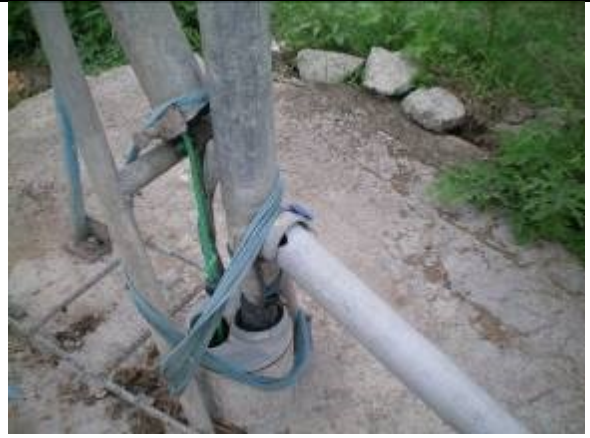
Return pipe not sealed, PVC parts broken, Pipe end cap is cut and has large holes so water leaks back in well.
