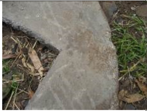
The manhole makes the well cover weak. Like in this case there is a crack cracked in the corner so another source for leaking water in the well.
