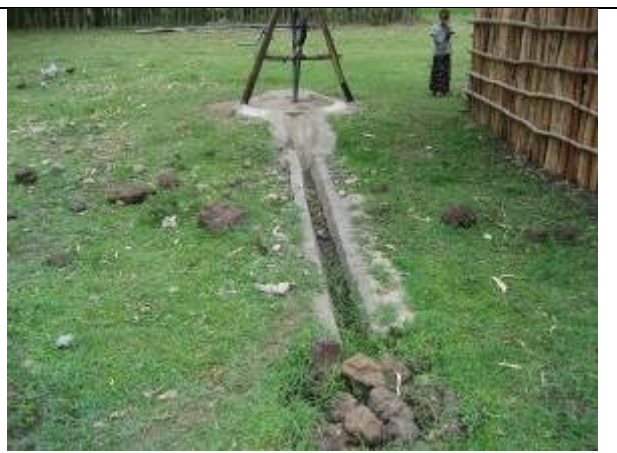
Good example of Soakpit, all water goes to the pit. The pit is filled with stones so no water is visible so not drinking of cows, no mosquitos etc.
