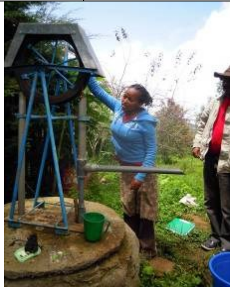
Pump high since it is mounted on a parapet. In this case short base model should have been used or a platform should be installed.
