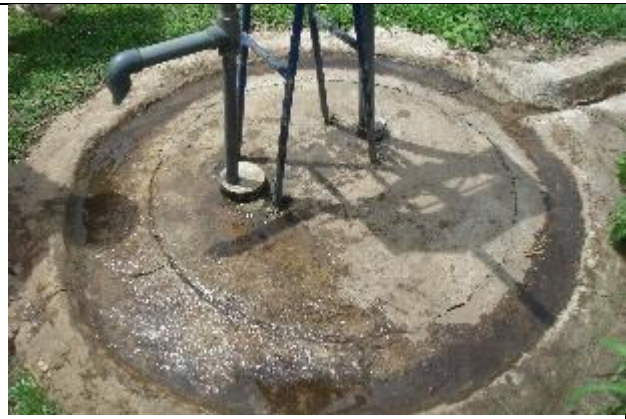
Here the well slab is not sealed well on the well rim.
