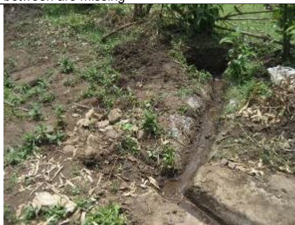
Bad example of Soakpit, The pit with stones was blocked and a new hole for cattle was made. This results in contaminated water.
