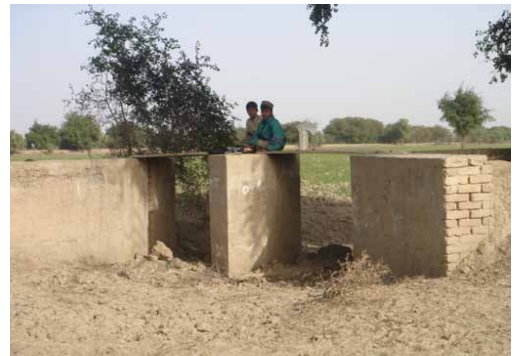
Figure 5: Large field bunds in spate irrigation developed by co-owning tenants (Photo credit: MetaMeta)
