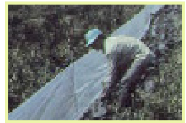
Figure 50: Installing the plastic fence of a Trap Barrier System with the cage inside at the fence; this TBS now awaits planting of traps crop and construction of moat around the outside perimeter.
