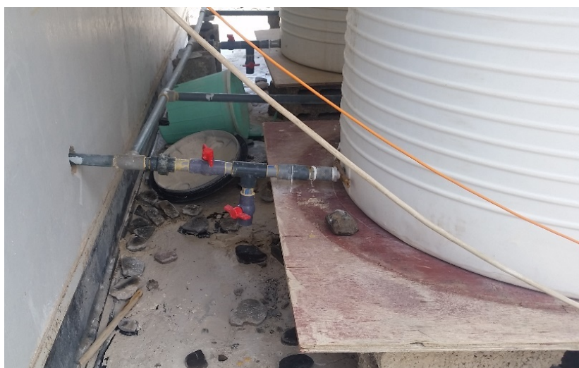
Figure 4: Calcium hypochlorite unit at main reservoir
